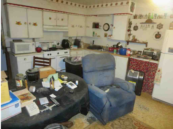
Kitchen Deteriorating Flooring
