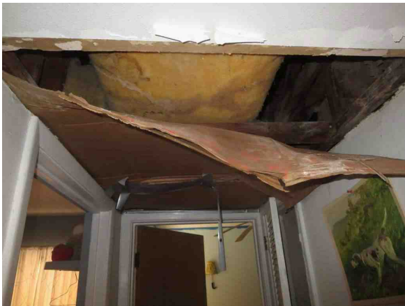
Evidence of Possible Water Damage from defective roof on Hallway ceiling 1 of 2
