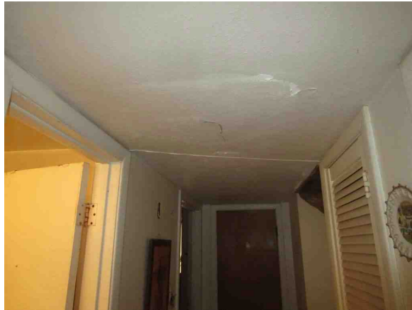
Evidence of Possible Water Damage from defective roof on Hallway ceiling 1 of 2
