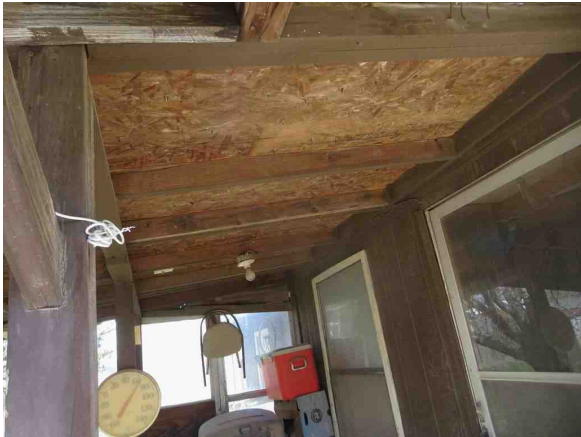
View of Covered Patio Does not appear to be weatherized
