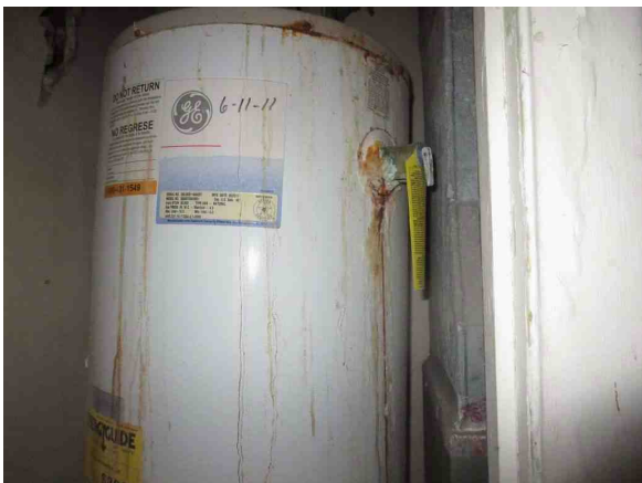
Corrosive/Defective/Deteriorating Water Heater Possible Safety Hazard
