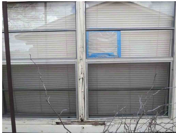
Sampling of Defective/Deteriorating Wooden Window Trim Broken Window Pane
