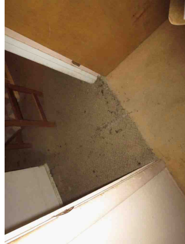
Sampling of Defective/Deteriorating flooring
