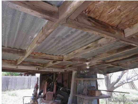
View of Addition Cover Connected to Covered Patio Appears to be Defective and not structurally sound Possible Safety Issue
