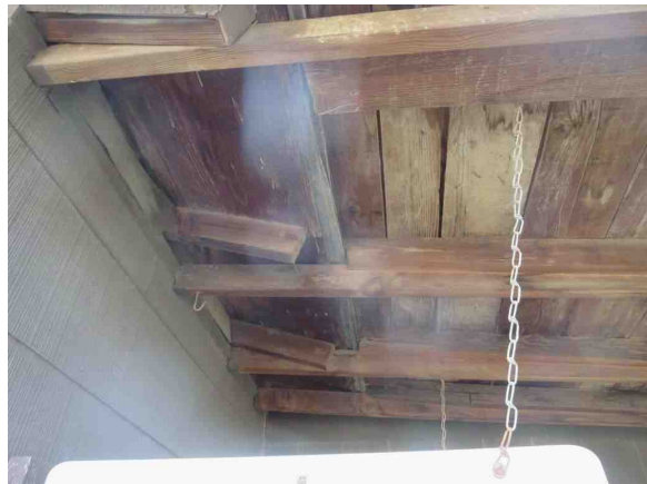
View of Covered Patio on Right Rear 2 of 3 Possible Safety Issue/Appears to be Structurally unsound
