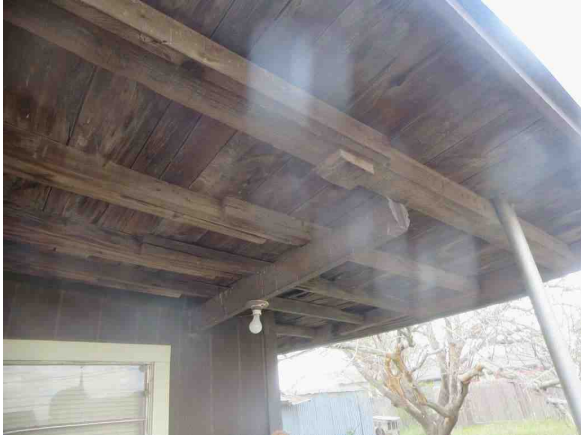
View of Covered Patio on Right Rear 3 of 3 Possible Safety Issue/Appears to be Structurally unsound
