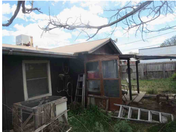
View of Missing/Defective Roof on Rear
