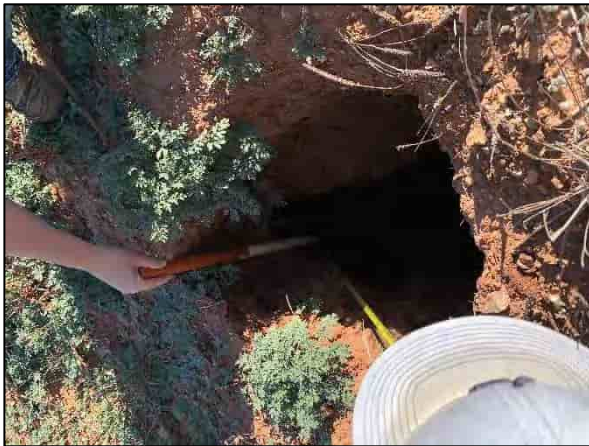
Large hole resulting from longitudinal cracking. (10/2020)
